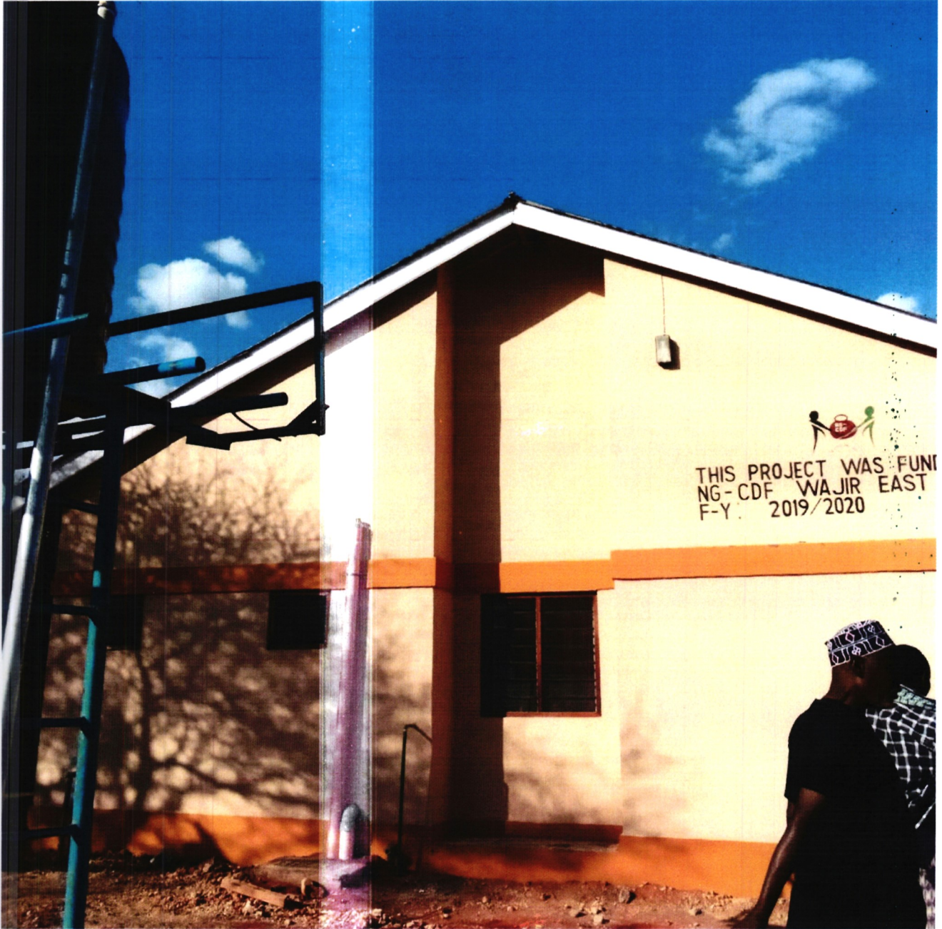
The Construction of Khorofharar sub county deputy county commissioner's residence at khorofharar town for the Financial Year 2019/2020.
