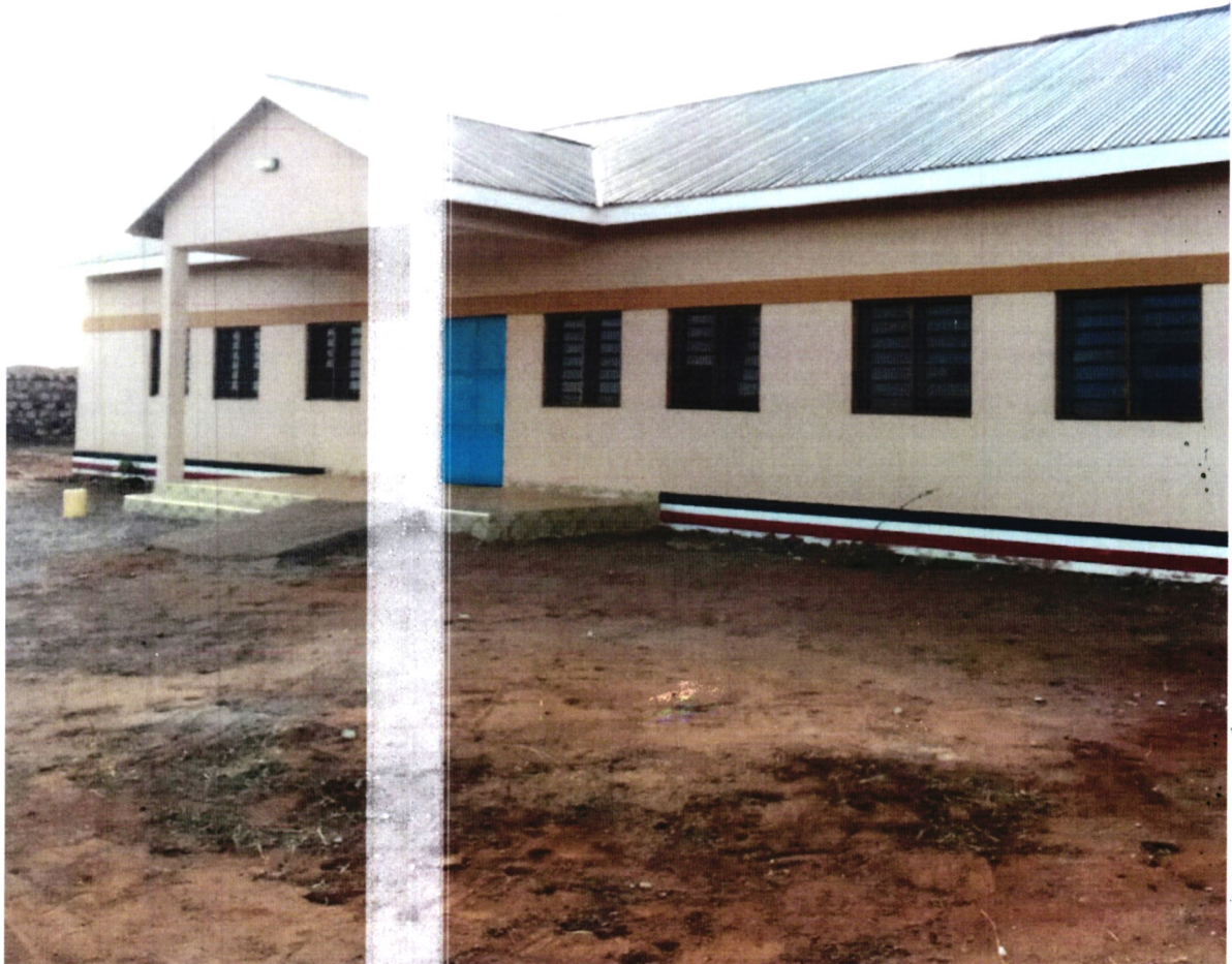
The construction of the Khorofharar Sub county deputy county commissioners office at Khorofharar town finanacial year 2019/2020
