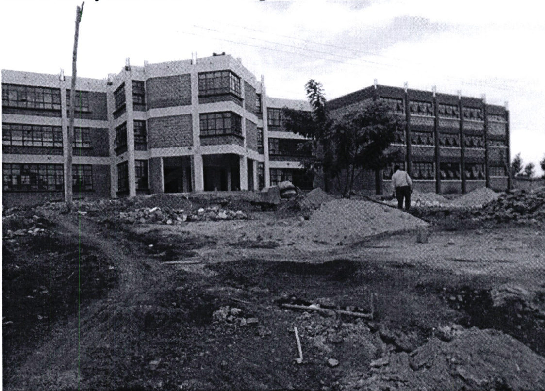
Pic. 1: Administration offices and classroom complex at Moi Girls High School - Vokoli funded by Sabatia NG-CDF
