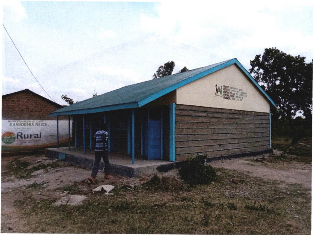
Figure 3: Completed Classroom at Kanyodera Pri. School which has helped in decongesting classes
