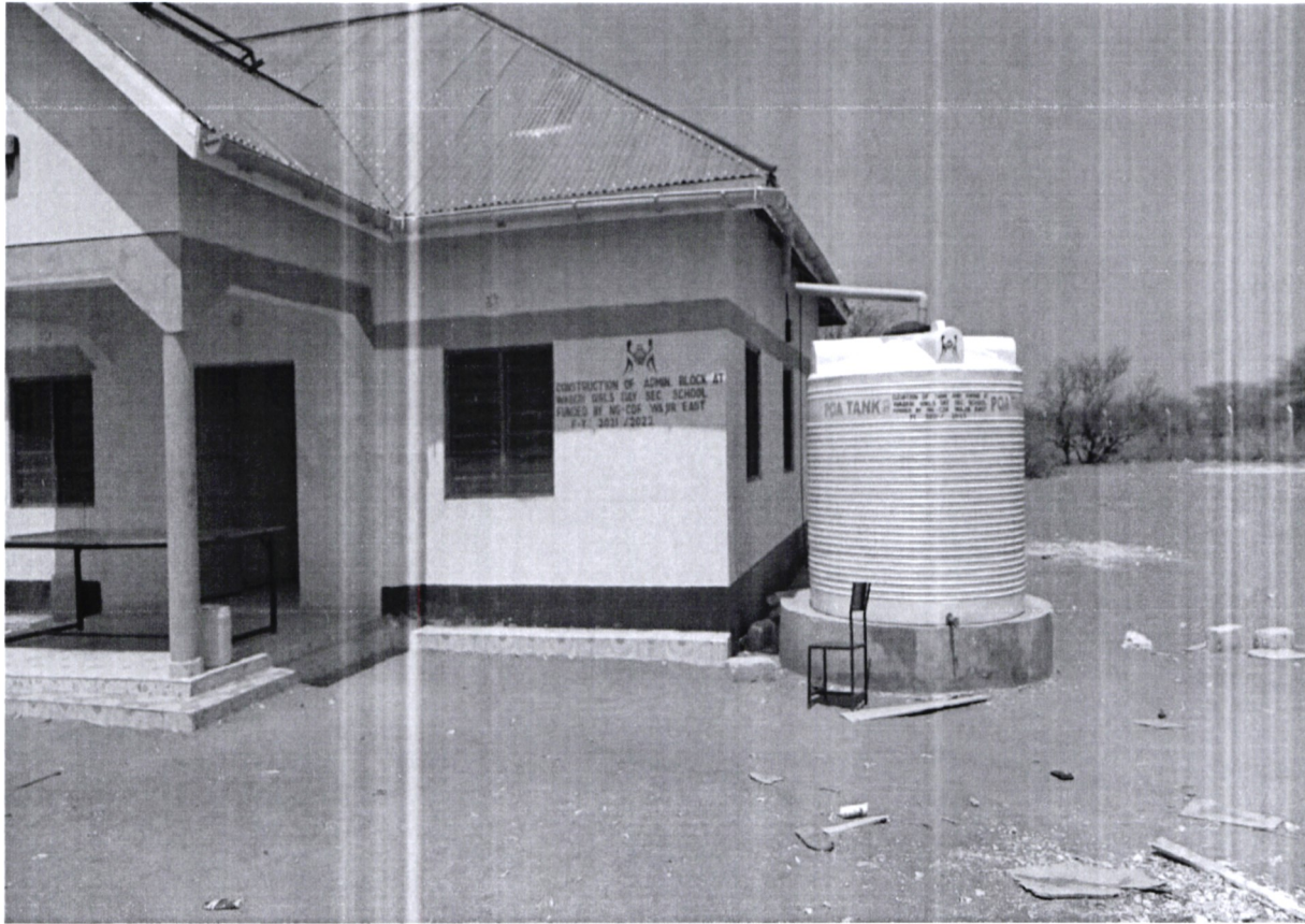
Waberi Girls Secondary School FY 2021/2022 Construction of administration block/supply and installation of water tank and water piping system
