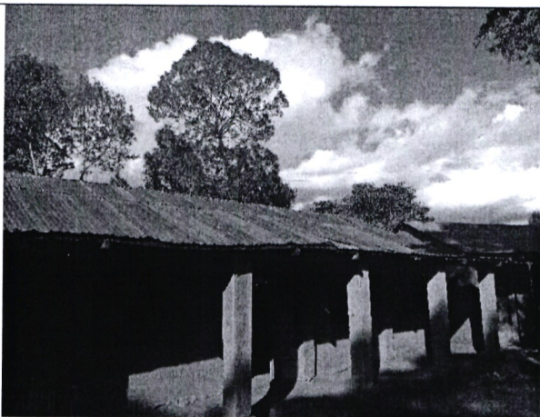
NGONDA PRIMARY SCHOOL. RENOVATION OF 8 CLASSROOMS(BEFORE)
