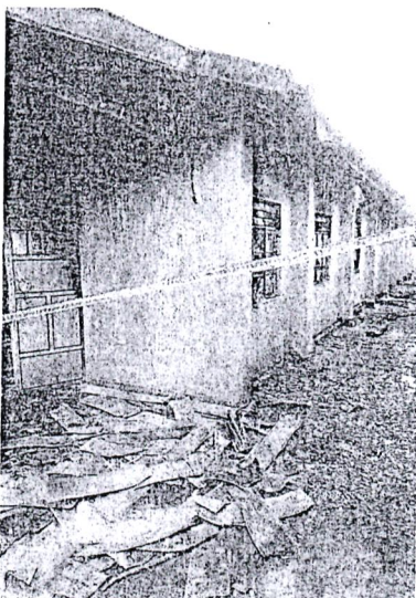
A dormitory destroyed by fire at Maranda High School /DICKENS WASONGA
