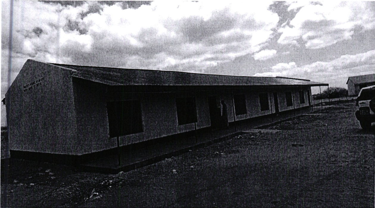
Construction of three classrooms at Salalama Primary School. This is one of most populous and best performing school in the constituency. Three classrooms enhanced the quality education by decongesting the students per classroom.
