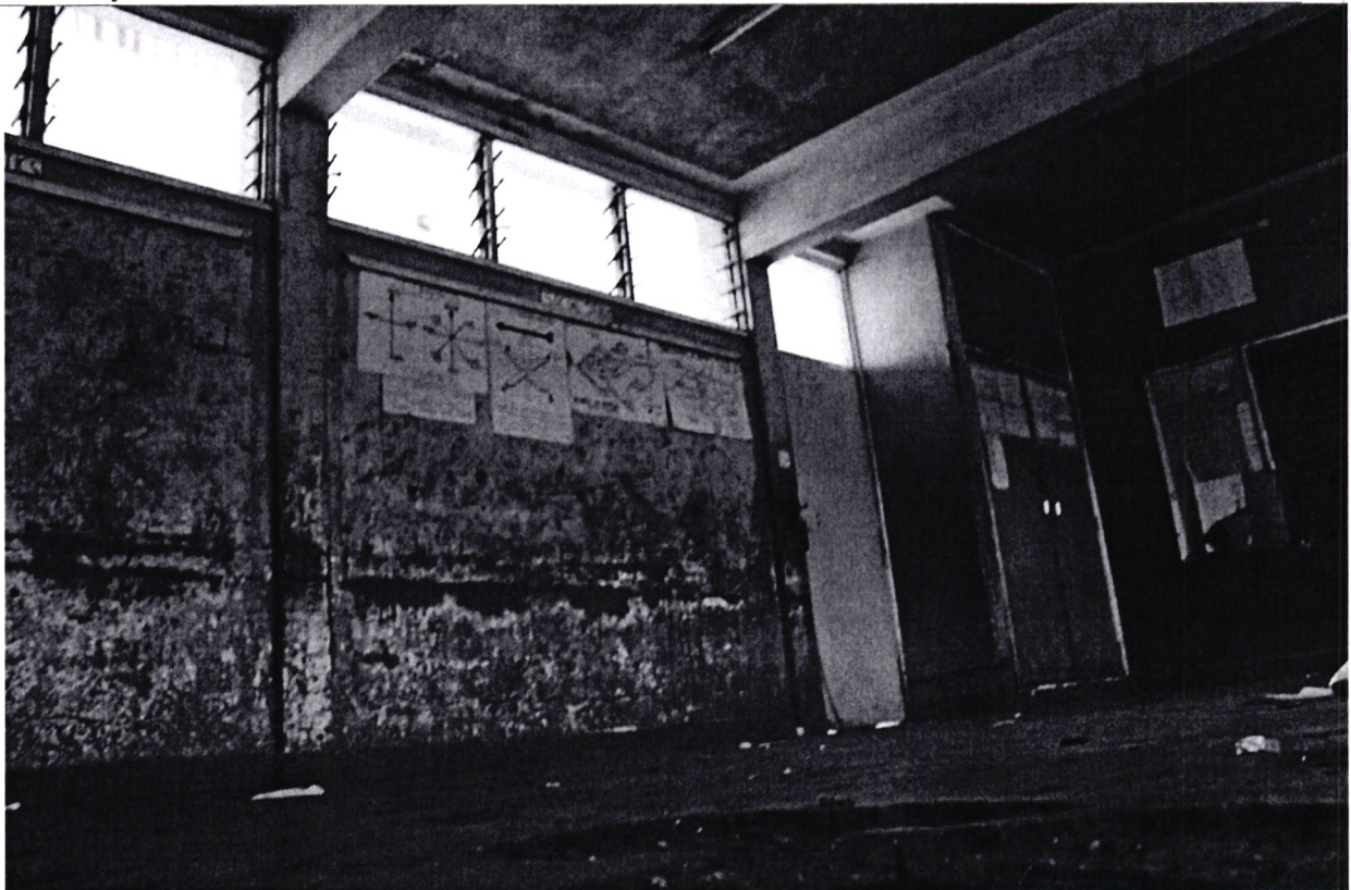
Madaraka Primary School – Before renovation
