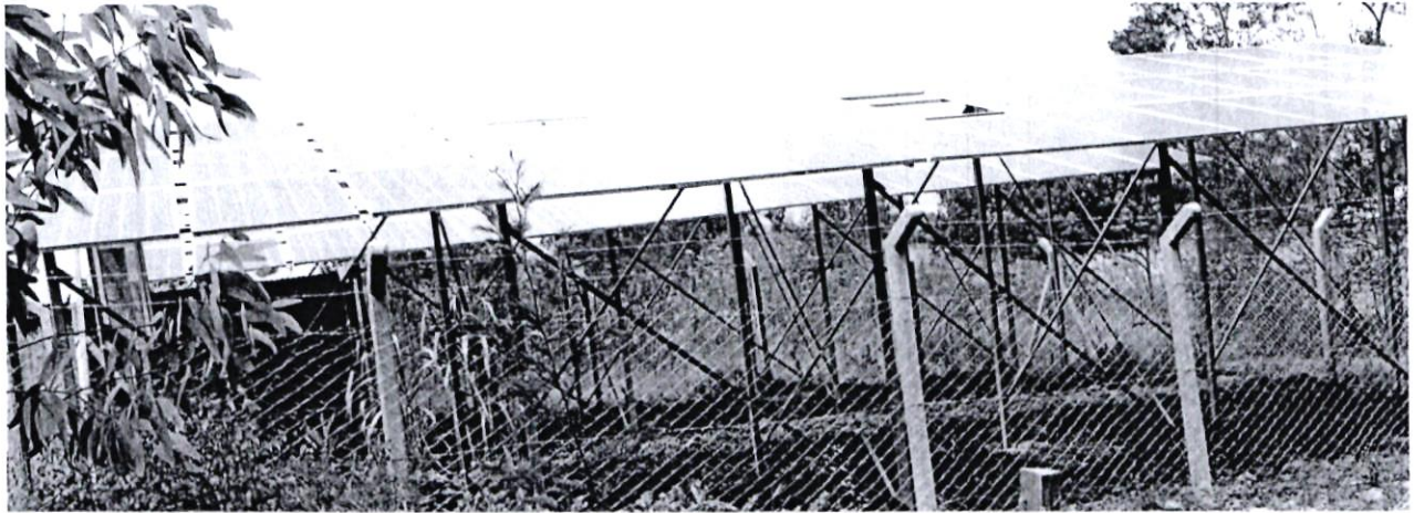
Ongoing Mutoigu intake at Gura River in Aberdare forest
