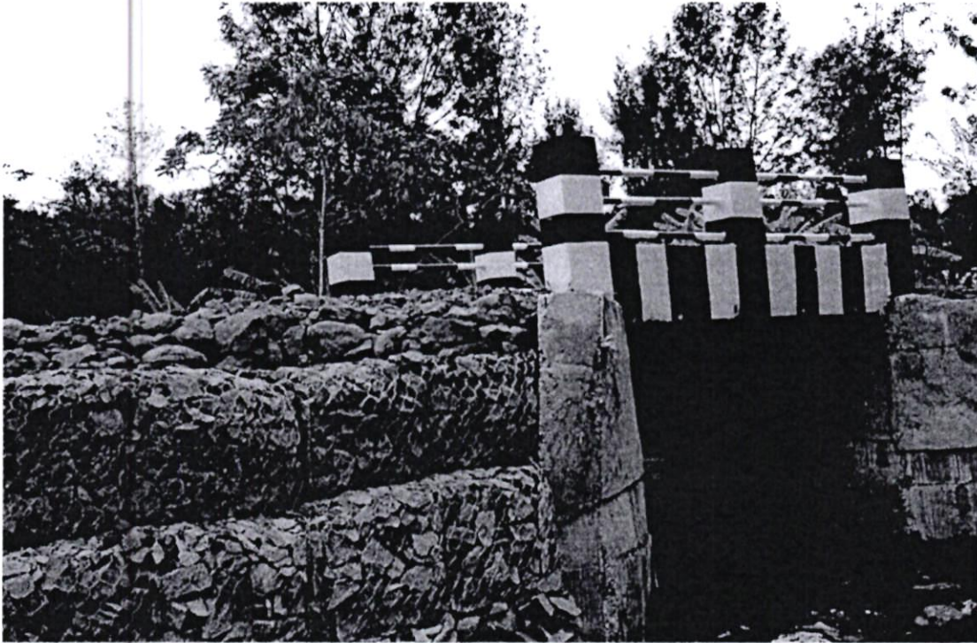
Gitegi – Kamweiga box culvert near Nyaribo township at Kiganjo/ Mathari ward, Nyeri Central sub-county is now complete.
