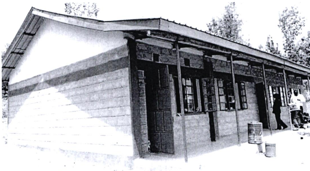
Classrooms have been constructed at Hiriga ECDE Center in Ruguru ward, Mathira West Sub-County.
