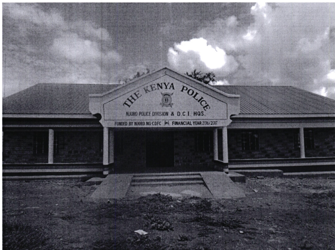
FIG 1.2 Construction of an OCPD Njoro office to improve service delivery at the Njoro Sub County. The office also has Criminal Investigation Department and the Deputy OCPD offices.
