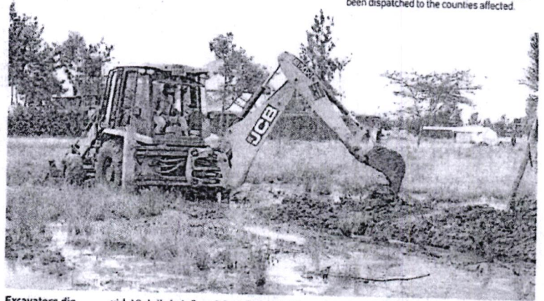
Excavators dig trenches at Mugutha village in Juja, Kiambu county. Residents are racing against time to clear waterways. PD/ MATHWU NDUNGU
