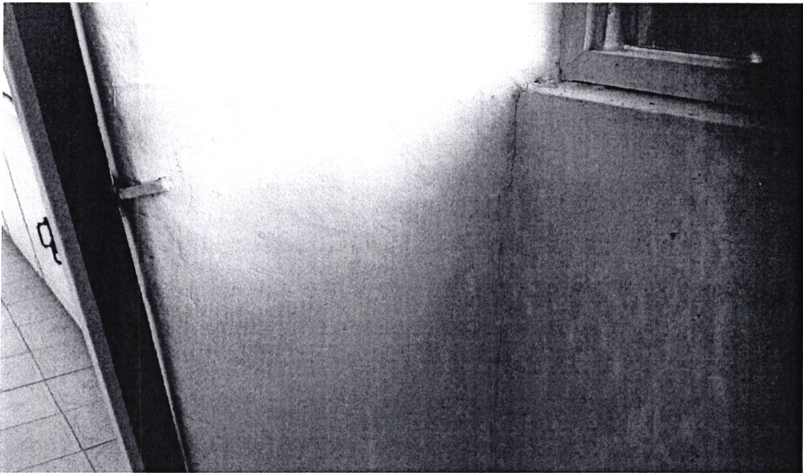
A minor vertical crack on one of the walls (the crack does not pose any structural challenge)
