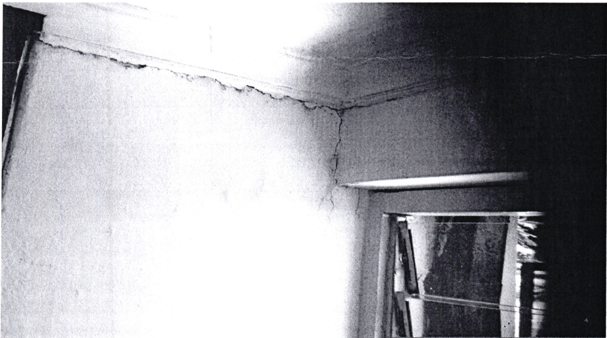
A minor horizontal crack on one of the walls (the crack does not pose any structural challenge)
