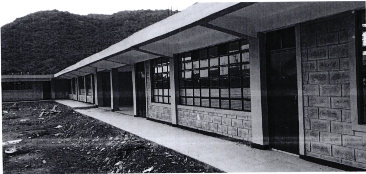
On-going three (3no) storey building at St. Triza Mundere Girls Secondary School
