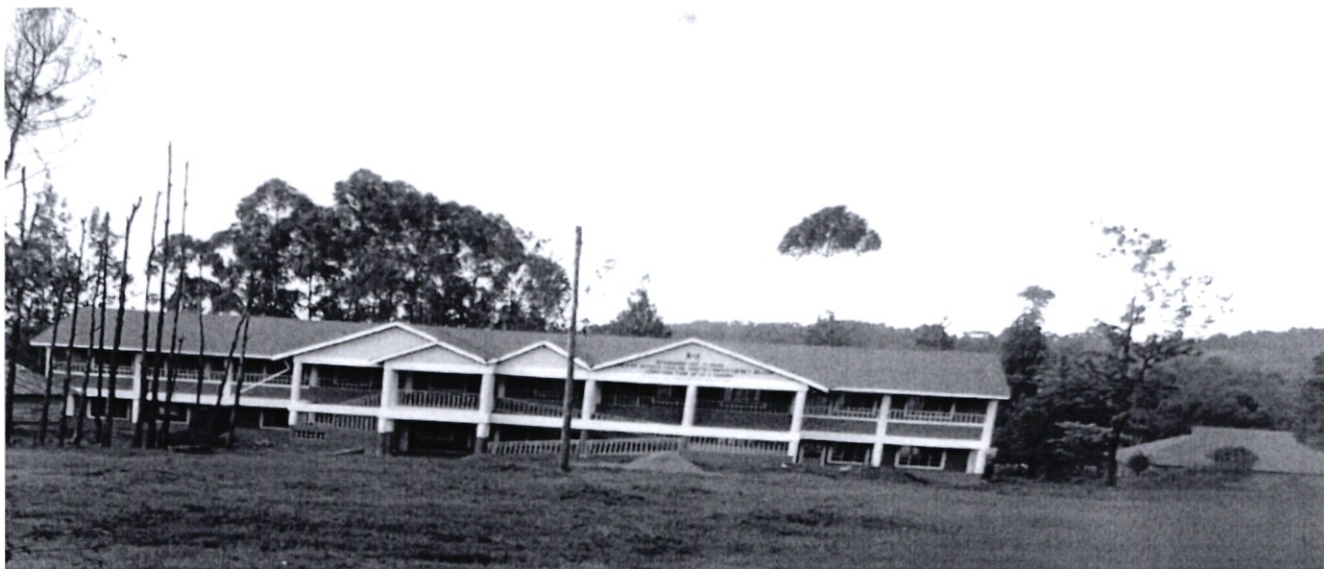
KITUTU CHACHE SOUTH NG CDF PROJECT-10 CLASSROOMS CONSTRUCTED BY NG-CDF AT NYANGURU SECONDARY SCHOOL
