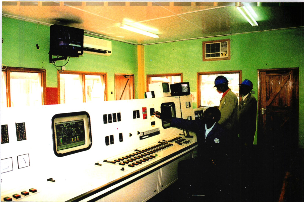
Computerized Control Room for the Diffuser at Mumias Factory
