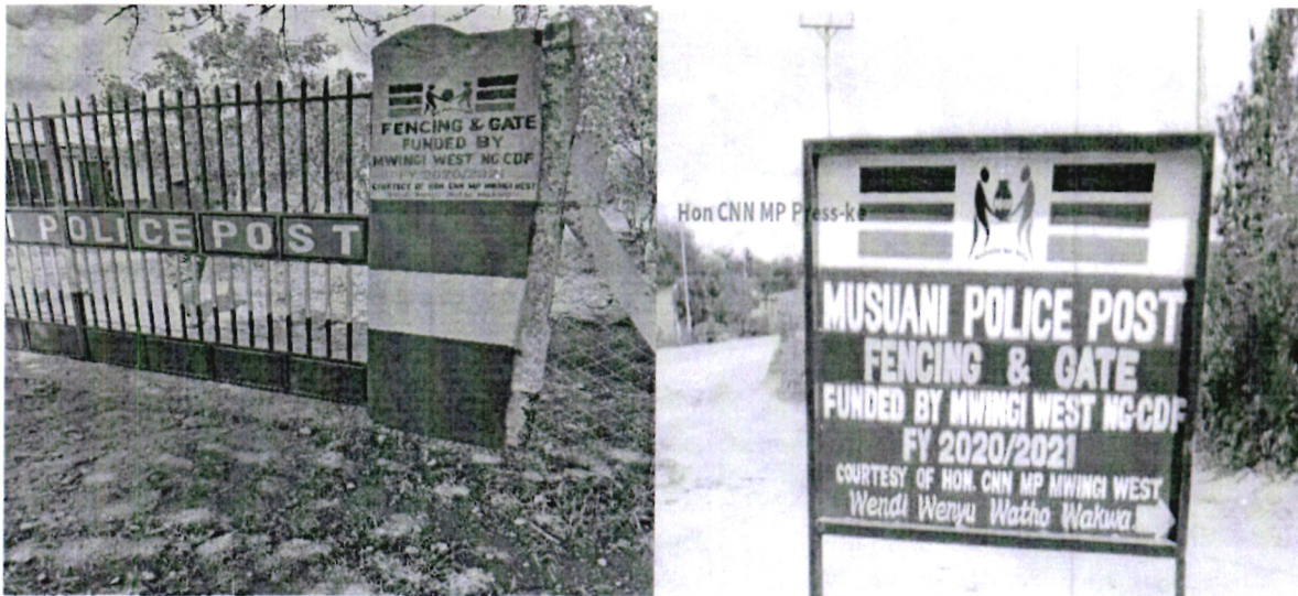
FIG 1.3: Fenced and installed a gate at Musuani Police Post FY 2020/2021, to enhance security and working environment to the officers.
