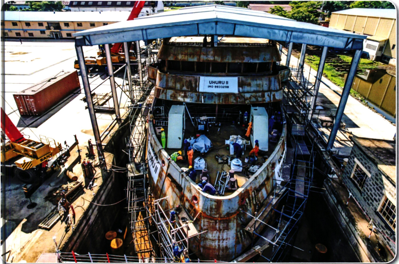
Ongoing construction of the first Kenyan-made Ship, MV Uhuru II, at the Kisumu Shipyard as at 30th June 2022
